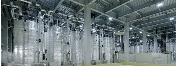
Example of indoor installation
