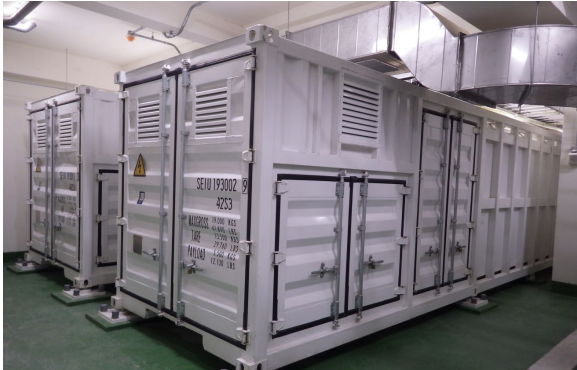
Example of underground installation
